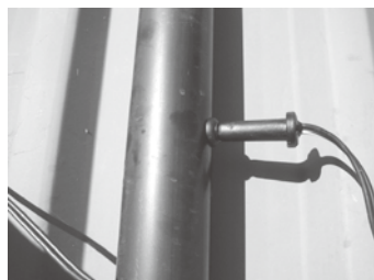
Figure 11: Rotoflow Probe Installation
